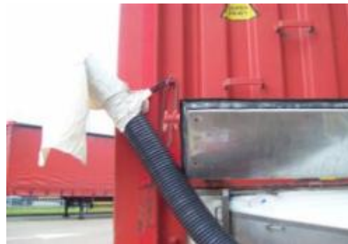
Vent pipe and vent bag
