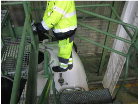
Fall restraint system not properly designed / Gaps which allow a worker to fall through
